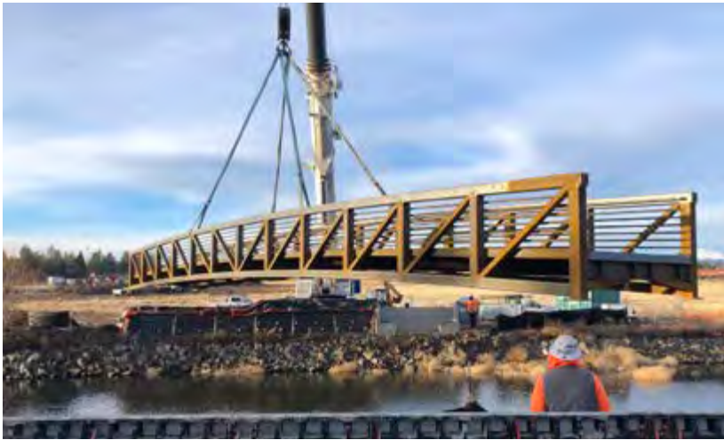
With construction underway at the future site of Alpenglow Park, BPRD crews and contractors placed a pedestrian bridge across a canal connecting a local neighborhood and providing traffic-free entrances into the park.
